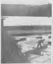
BEFORE CONSTRUCTION could start, the refinery site had to be elevated fifteen feet. accomplish this, 6,000,000 cubic yards of fill were hydraulically moved to the building by the municipality of Rotterdam.
